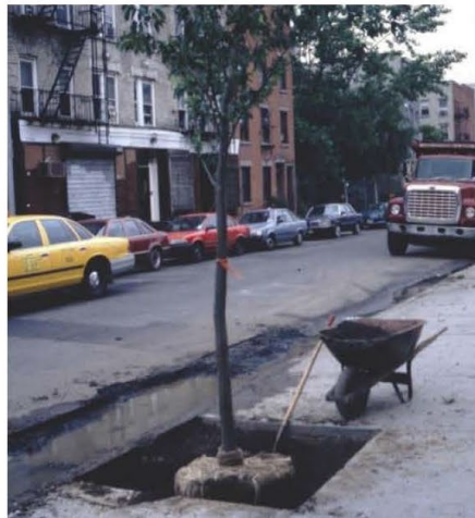
Standard City Tree Pit Inadequate Conditions for Tree Health
